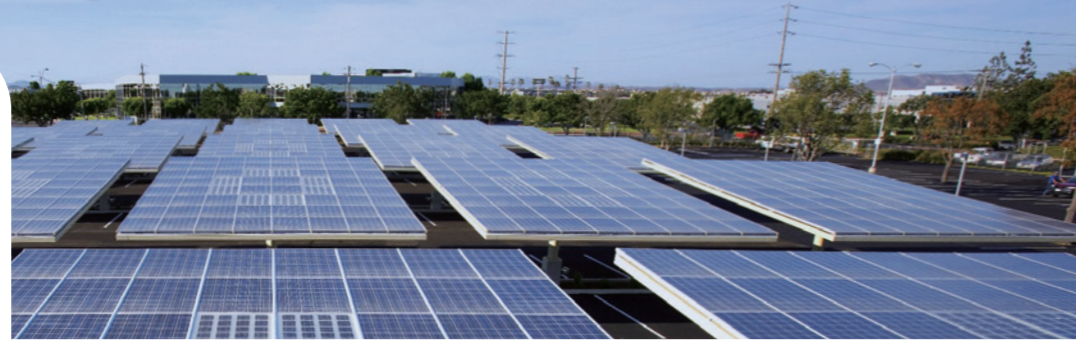
Solar power generation facility using Bridgestone's adhesive film from photovoltaic modules
