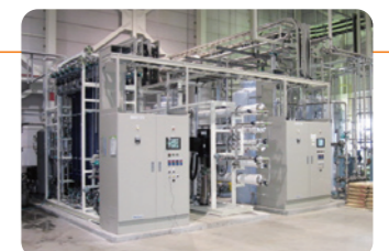
Water recycling system at Kitakyushu Plant (Japan)
