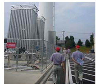
Natural gas tank in Bridgestone Iwata Plant
